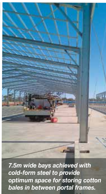
Mild steel columns and partially boxed rafters to eliminate knee bracing and meet the customers storage requirements.
